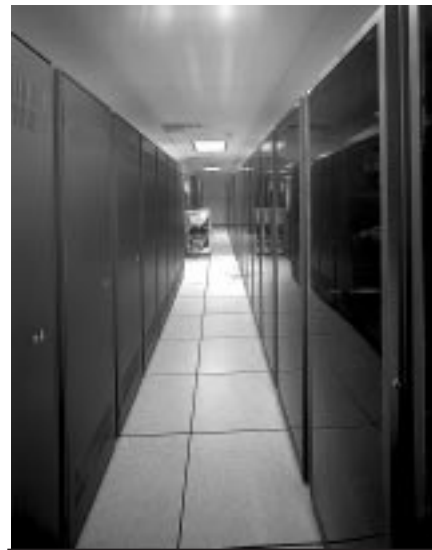
Management of hardware systems was established through cabinet environment and ensured system security.
